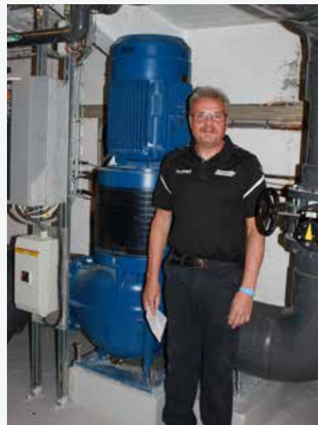
Tommy Pedersen, Technical Manager at Noerresundby Sports Center in front of the DESMI DSL 250-310/D-G pump, which pumps 620 cubic meters of water per hour.
